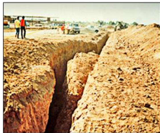
Figure 1 Excavation Cave In
